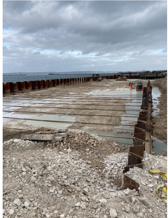
Figure 2: The Anker Schroeder tie rods
